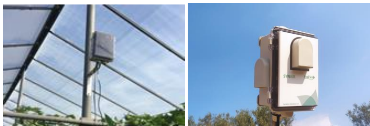
Figure 64: SynAir indoor (Greenhouse) and outdoor Installation
